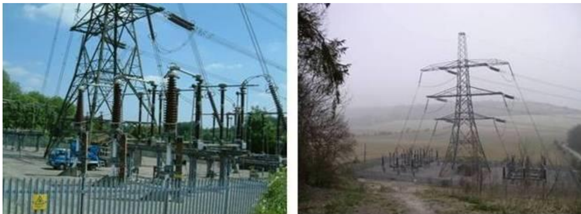
Figure C.5: Cable Sealing End Compounds
